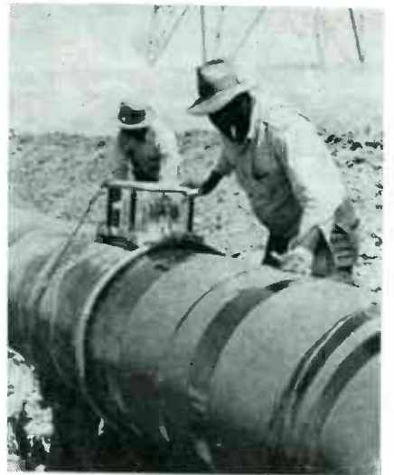
Operators use the high-voltage tester for finding weak spots in the coating of Biggest Inch, a gas pipeline of Southern California Gas Company
